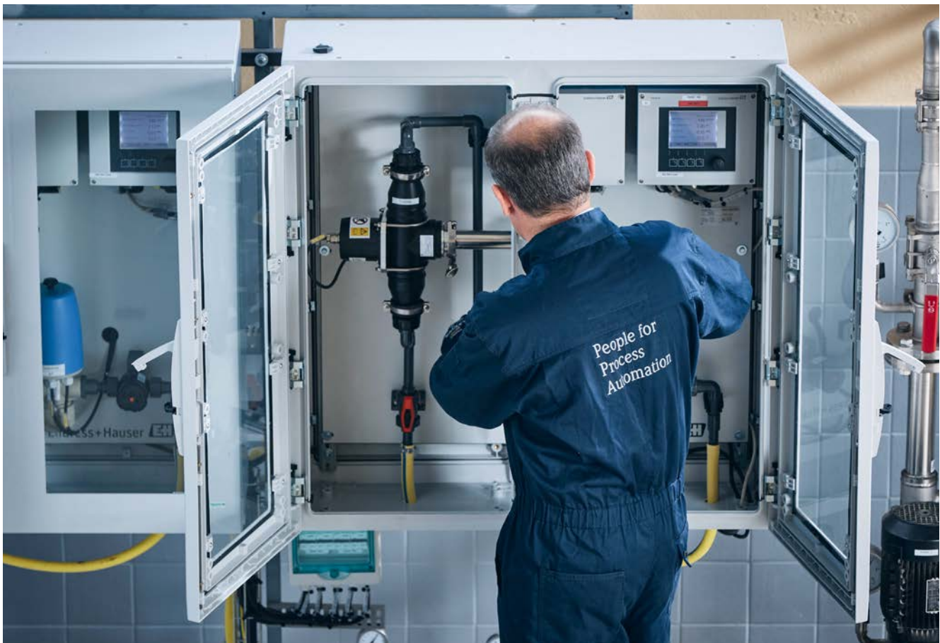
The measuring technology for Critical Control Points (CCPs) is often installed on a panel. A protective enclosure is also sometimes used to protect the measuring technology. Our service engineers will be happy to help you install and maintain your CCPs.
