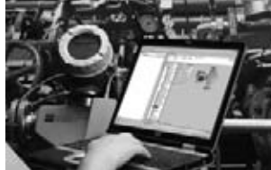
Commissioning and configuration with FieldCare
