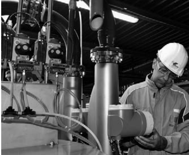
Flowmeters connected to a PROFIBUS network
