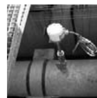
Air injection regulation in the pond of aeration (wastewater)
