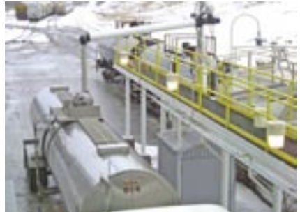
Railcar filling of water treatment chemical using mass flowmeters
