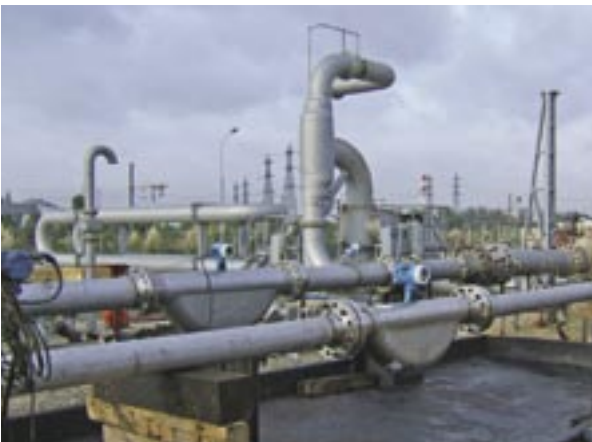
6" and 10" Coriolis mass flowmeters installed in gas pipe application - no additional brackets or supports required
