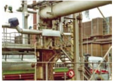
Truck loading of chemicals using Promass M mass flow measurement
