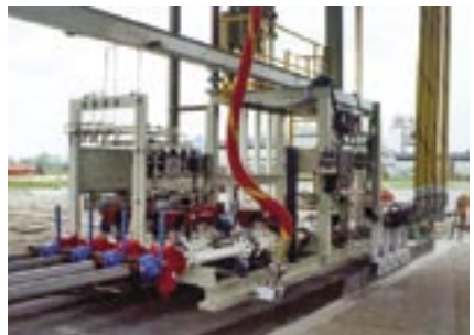
Petroleum truck loading application using mass flowmeters in conjunction with Coriolis for custody transfer verification
