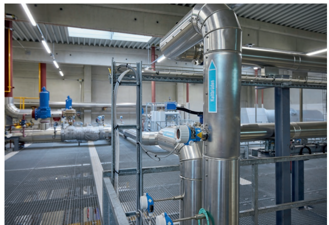
In the new boiler house, where vapor water from the spray drying tower is converted back into steam, numerous instruments from Endress+Hauser monitor the processes.
