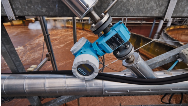
Proline Promag W50 electromagnetic flowmeters for aeration of the three activation tanks.
