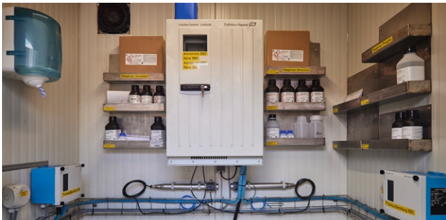
Complete monitoring of the activation tanks: ammonium and phosphate analyzers, as well as UV photometric measurement of nitrate with sample preparation.
