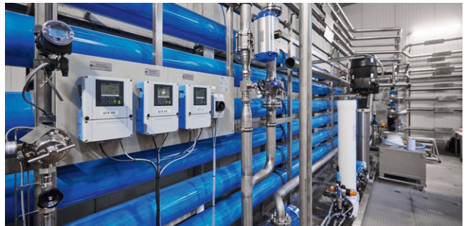
Reverse osmosis for producing process water, including conductivity and redox measurements.
