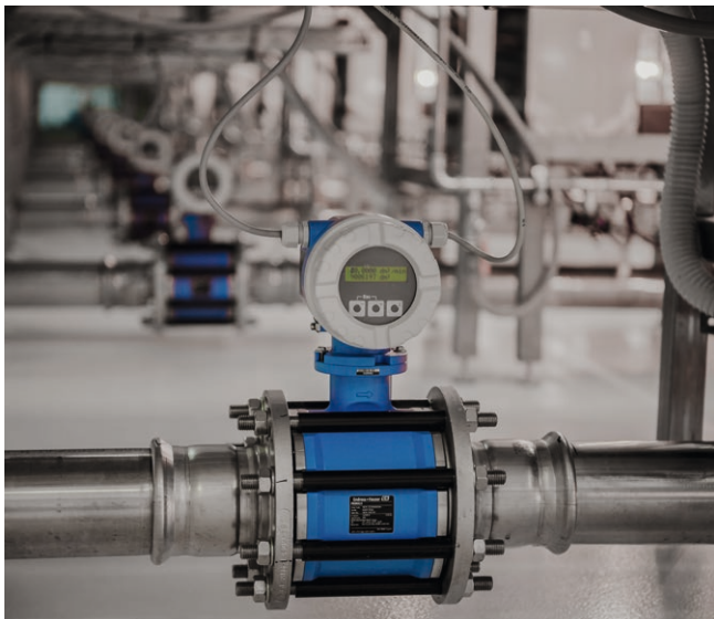
The Promag 10D electromagnetic flowmeter monitors the speed of the algae suspension as it circulates through the system.
