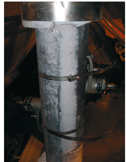
Prosonic 93P sensors mounted on condensate line
