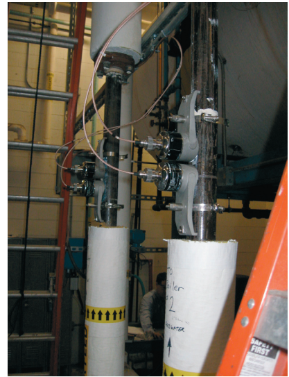
Prosonic 93P sensors mounted on water inlet piping
